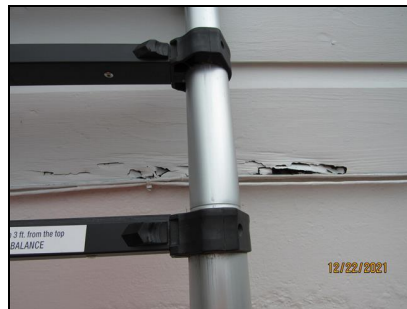
3.4 Item 2(Picture) Bottom of lap siding - left side
