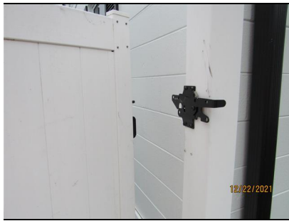
12.11 Item 1(Picture) Right gate not self latching
