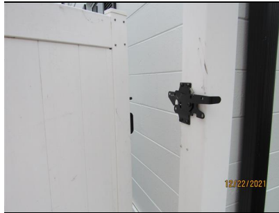
12.11 Item 1(Picture) Right gate not self latching
