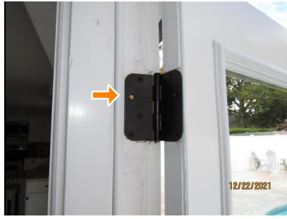
3.1 Item 3(Picture) Missing screw
