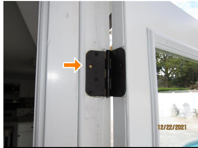
3.1 Item 3(Picture) Missing screw
